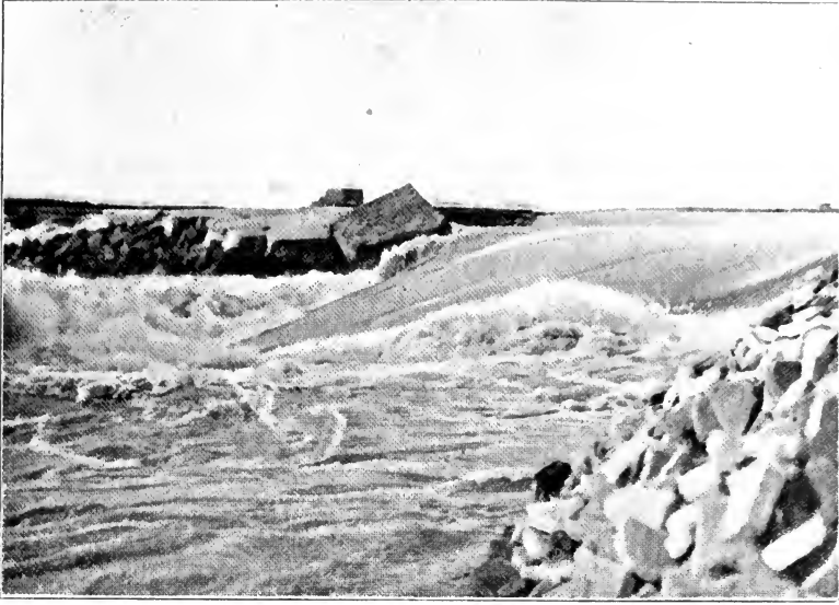
Breach in old Hindia Barrage on the Euphrates (from Downstream).
